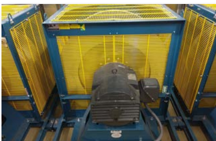
Model EPFN Supply Air Fans in Air Handling Unit
