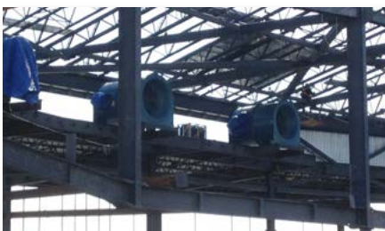
Model QSLSH Smoke Control - Amphitheater
